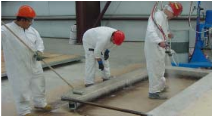
An initial coating shall be applied to all wall & roof sections, prior to erection of the Shelter
