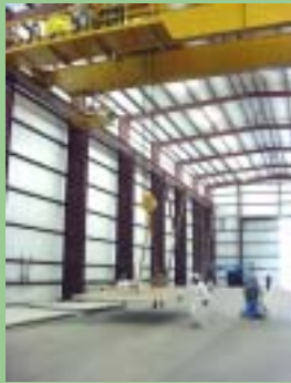
A 40 Ton Bridge Crane handles all the heavy lifting tasks
