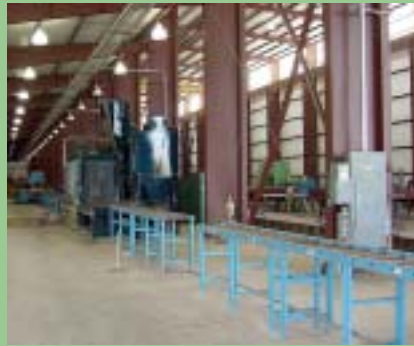
A Bead Blasting Unit is positioned in-line with a Cut-Off Saw to prepare all structural beams
